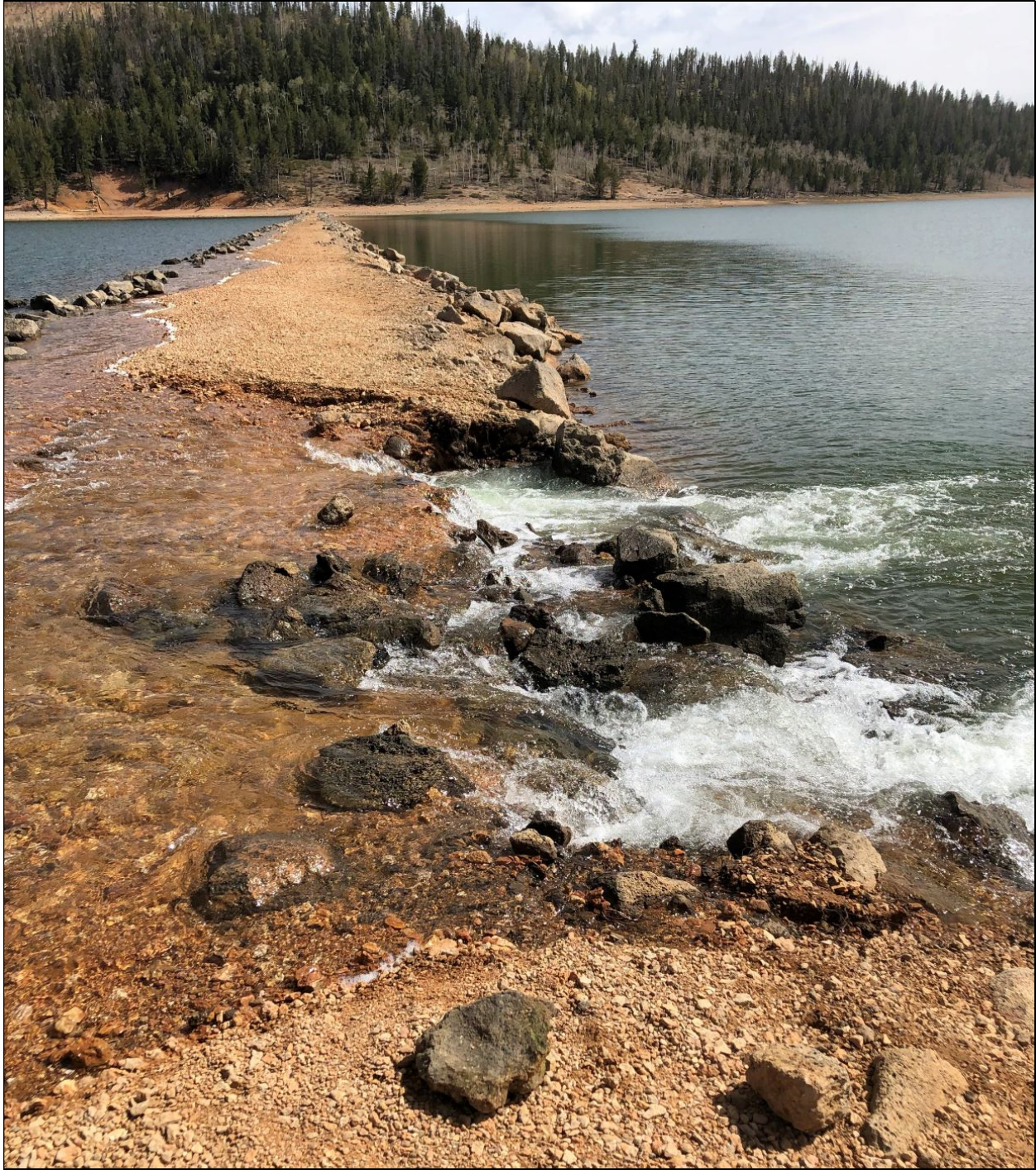
Figure 7. Erosion of the Navajo Lake dike observed in May 2020.
